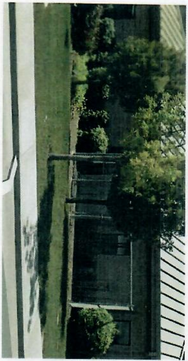
STREET VIEW OF SWITCHGEAR
